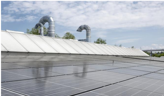
Photovoltaic solar panels
