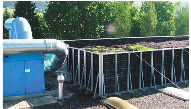
Biofilter plant on the factory roof
